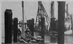
AS THE piles went in, carpenters installed pipe supports. CARPINTERAN a instala balhainan di dwars.
